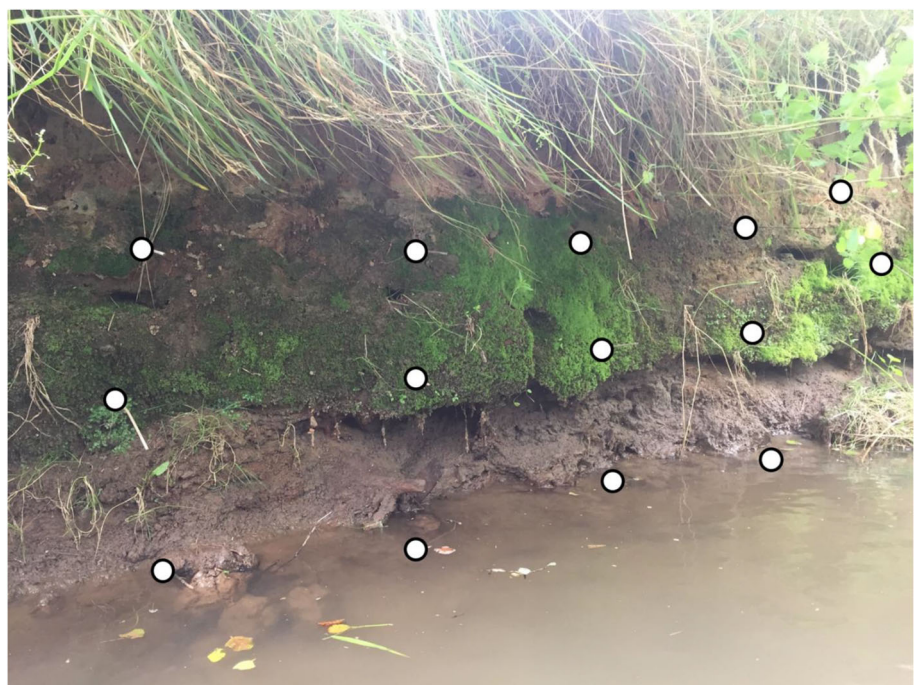
FIGURE 5 An undercut bank on the River Bain. The spacing of the erosion pins (denoted by circles) was often too coarse to detect these local processes which lead to large-scale collapses. (NB: Photograph taken during low flow conditions for clarity of bank morphology)
