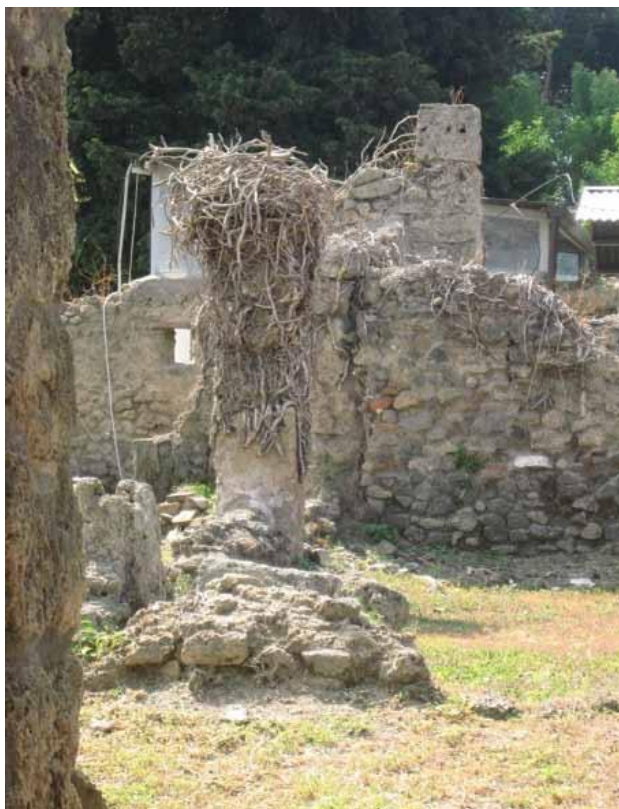
Figure 42. Overgrown vegetation and crumbling walls in an unvisited area of the site, Thompson (2007)
